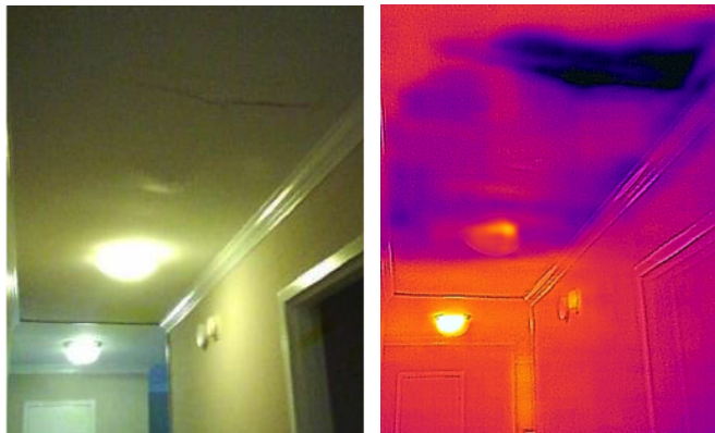
Figure 1: A participant found a water leakage problem when investigating a small drip on the wall. The thermal image revealed that the problem was much more severe than what was visible to the naked eye [5]
